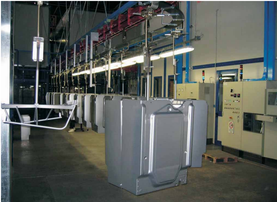
Figure 1: Transport line, one of the autonomously automated modules in the new paint shop
